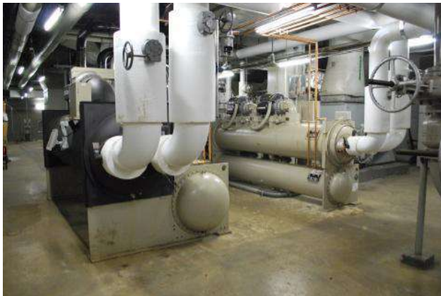
Chiller inside Tower's 1828 L St. Building
