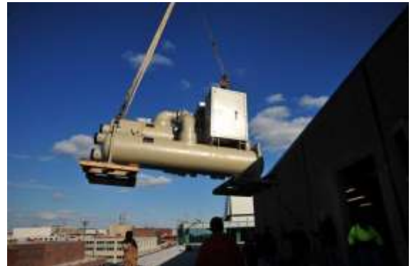
Frictionless centrifugal chiller installation
